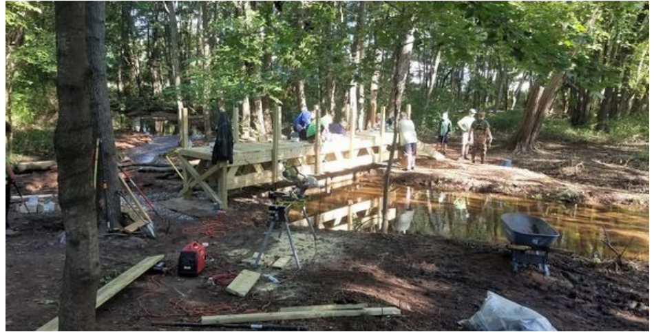
Stephen Gagnon, Eagle Scout candidate from Troop 27 in Manchester, worked on this 50-foot bridge at Salter’s Pond in October, 2021, with help from fellow Scouts, parents, and Land Trust stewardship chair Jeff Sullivan. The public and our neighbors at the Salter’s loop trail, Northfield Green Condominiums, chipped in $3000 for the materials. Jeff notes these other Eagle projects: • Conor Mulligan, Troop 123, trail at Barlow Park, Hillstown Road, January 2022, and • Ian Cameron, Troop 25, improvements at Salter’s Pond, March 2022.
