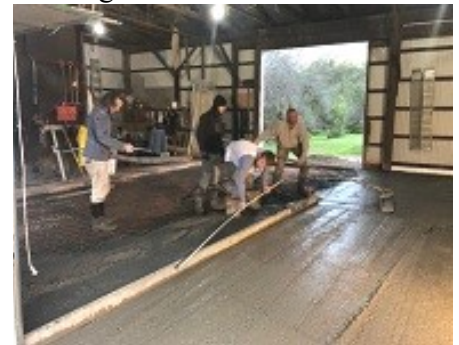
Above: pouring a solid floor at the red barn on our Bush Hill farm property, October 2018. Big job!
