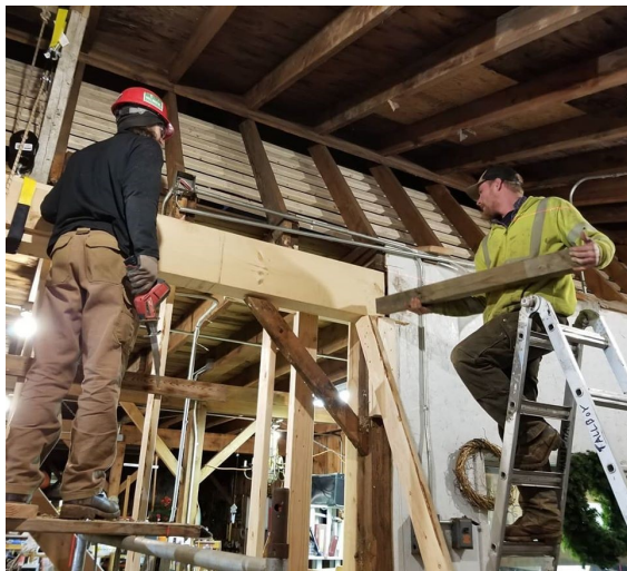
Barn beam replacement project, January 2021. The previous beam was water-damaged and disintegrating.
